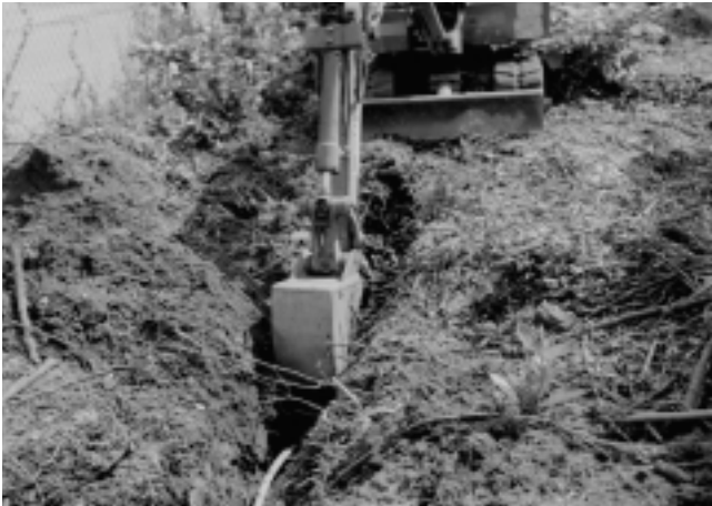
This cable jacket, damaged by an excavator, is quickly repaired.
